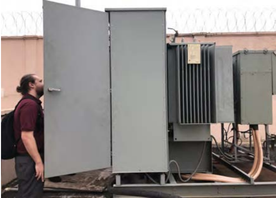
(b) An HV transformer
