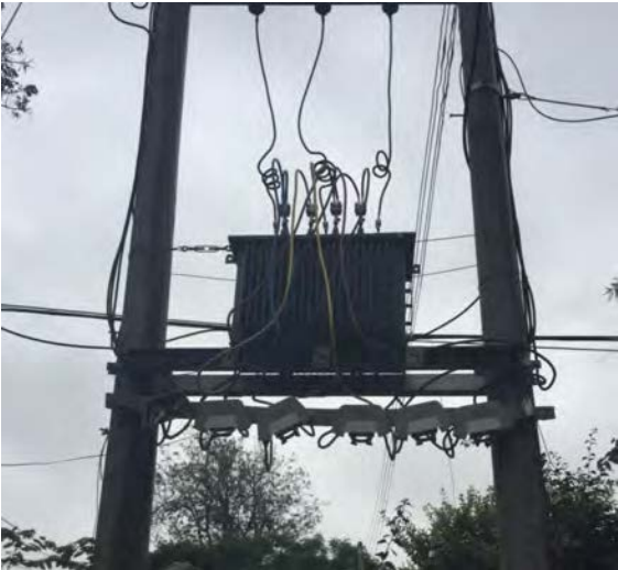
(c) A 3-phase LV transformer
