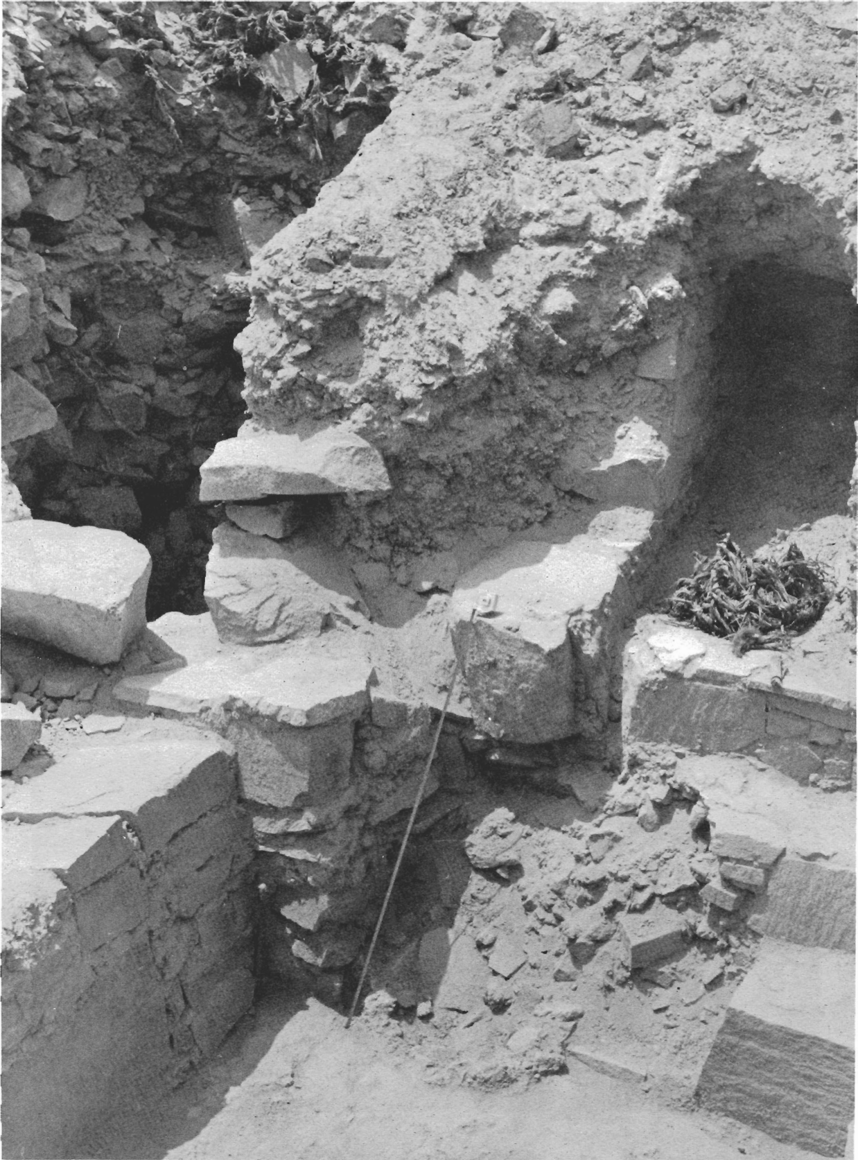
Plate XLIII. Fig. 9, Cut 5, showing the unfinished reconstruction of the stairway onto Structure 1 using concrete mortar. The mason's stake and string remain in the corner (lower left center). The stairs on the right were left incomplete; on the stair is a reed net for fill stones (right center). The tape shows 1 m.
