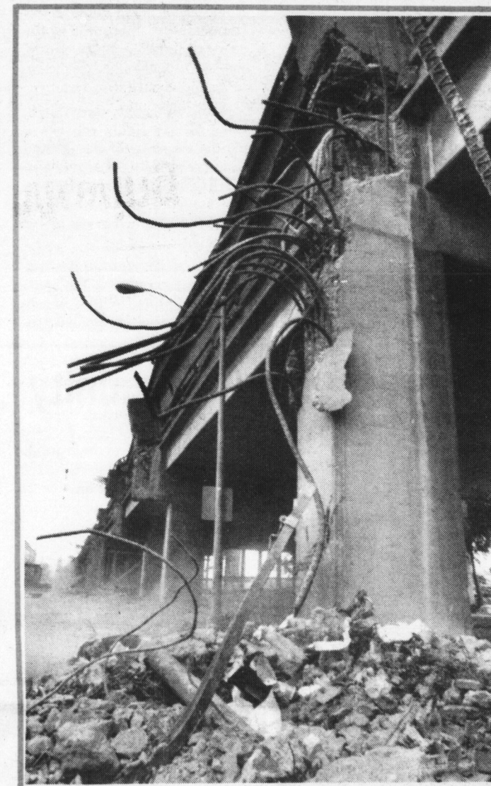
A portion of I-880, the Nimitz Freeway's Cypress Overpass, that collapsed during the earthquake that measured 7.1 on the Richter scale. (Photo: Rick Gerharter)
