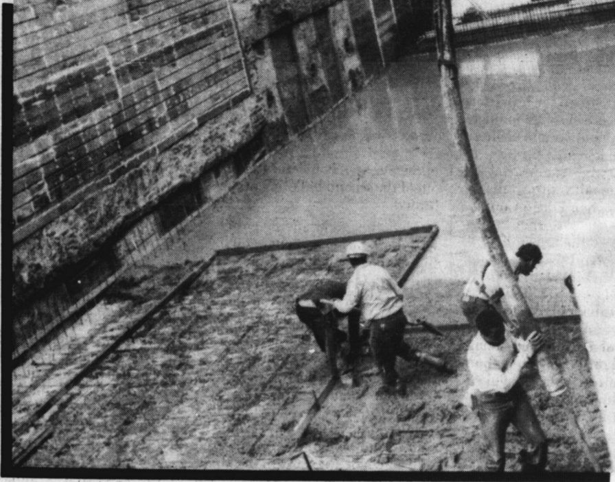
Workmen lay the foundation to the Atlas S & L building in the heart of the Castro. (Photo: Rink)
