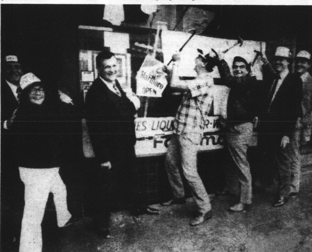
The Atlas Savings & Loan Board of Directors turned out in work clothes and hardhats to launch the demolition of the building at the site of the new branch on Castro Street. (Photo: Rink)
