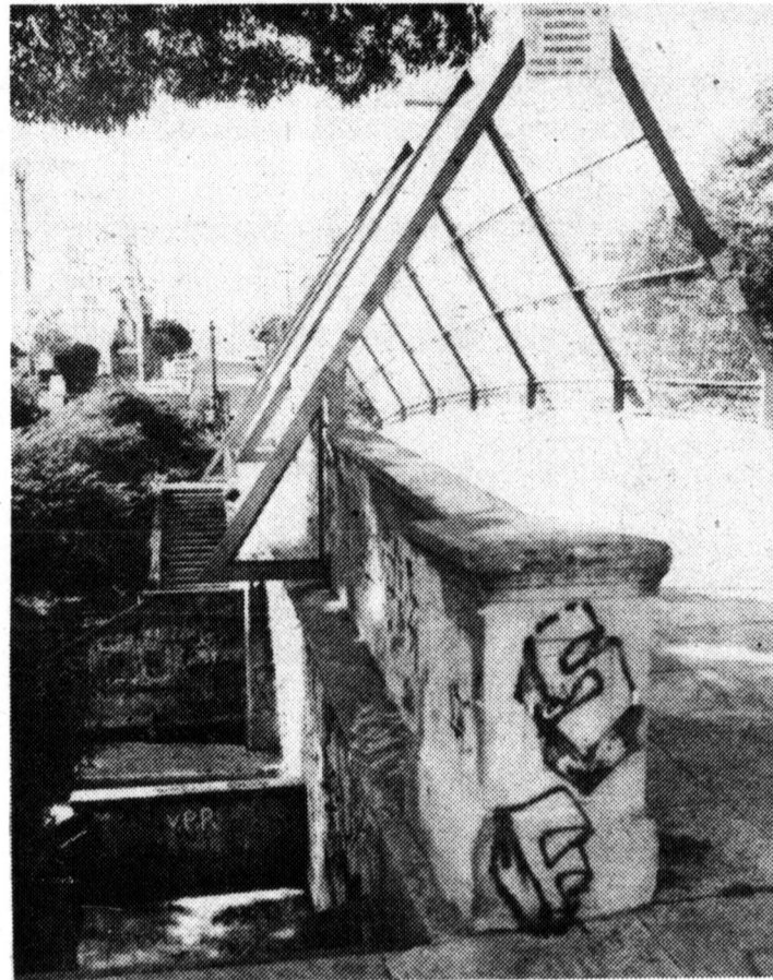
Dangerous Muni stop and overpass sports typical defacing graffiti. (Photo by Rink)
