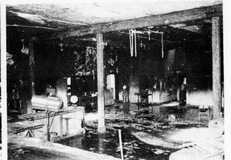
Some of the extensive damage to the Center.
